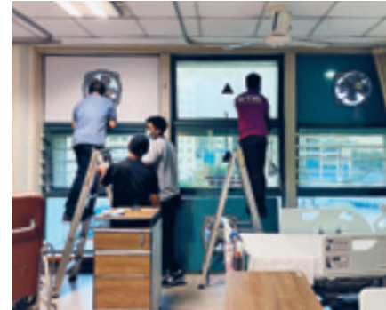
Below: The conversion of wards at TTSH Main Building to support COVID-19 care; Supporting NCID in scaling up bed capacity.
